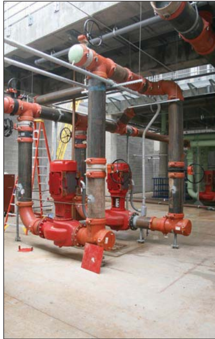
For the Methodist Sugar Land Hospital expansion project, MLN Company chose the Victaulic Advanced Groove System designed specifically for large-diameter piping systems, which it could install quickly and easily on piping connecting the pump and chillers to the rest of the system.
